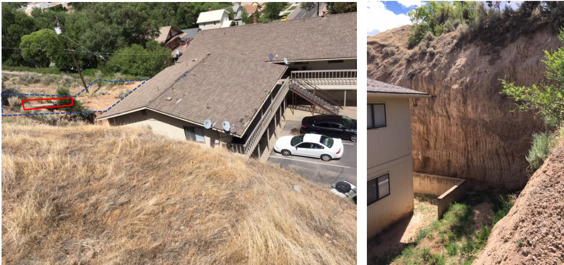
Figure 1: (Left) 235 Fravert Avenue Apartments from above, undermined storm drain circled in red and ROW denoted with dashed blue line (Right) Vertical excavation adjacent to apartments
