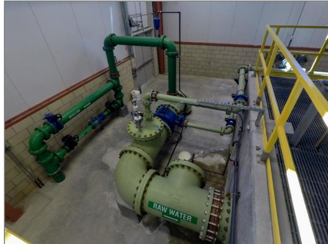
Pretreatment Chemical Injection and Jet Mixing Piping
