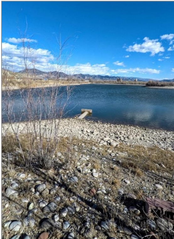
Raw Water Settling Pond Intake Pipe
