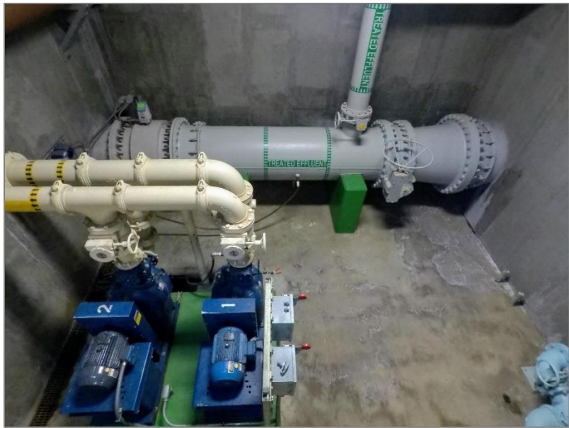
Treated Effluent Leaving the Disinfection Room
