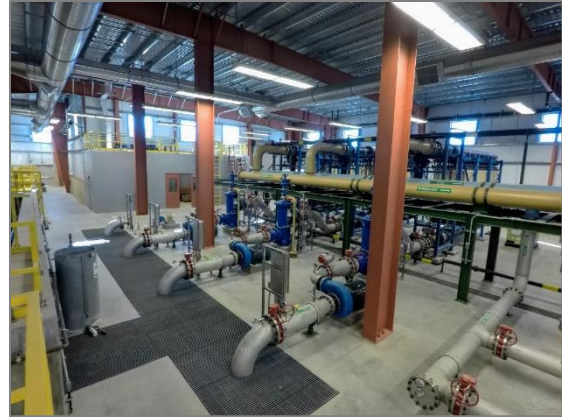
Pall Microza Membrane Filtration System
