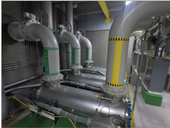
UV Disinfection Units
