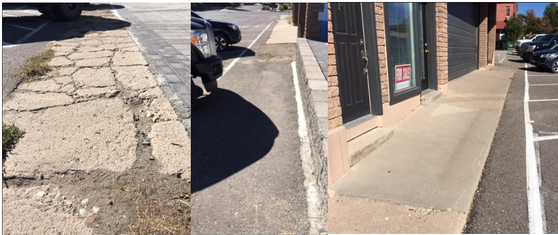
Figure 1. (Left) failed sidewalk on Second Street; (Middle) non-existent sidewalk on Second Street; (Right) Sidewalk with non-compliant cross slopes requiring steps into building access
