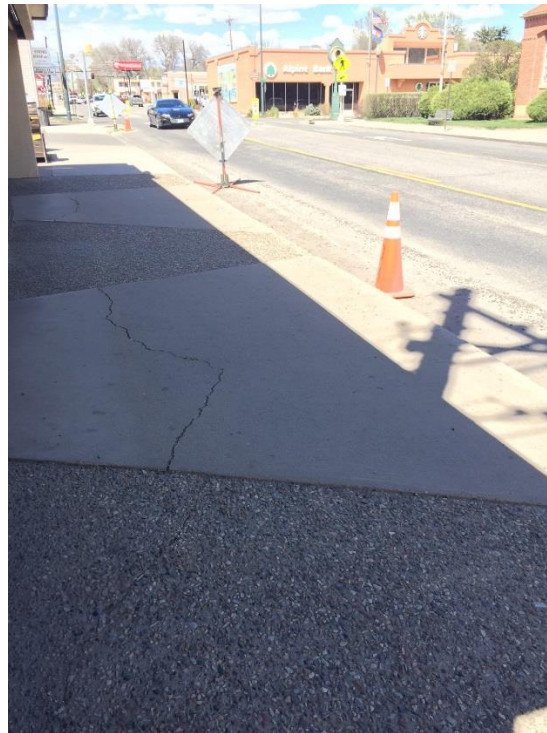
Photo 2 – Sidewalk Cracking in the 300-Block of Railroad Avenue, Looking South
