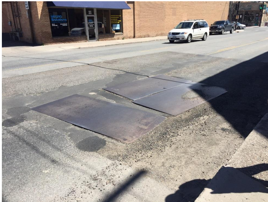
Photo 1 – Road Settlement in the 300-Block of Railroad Avenue, Looking South
