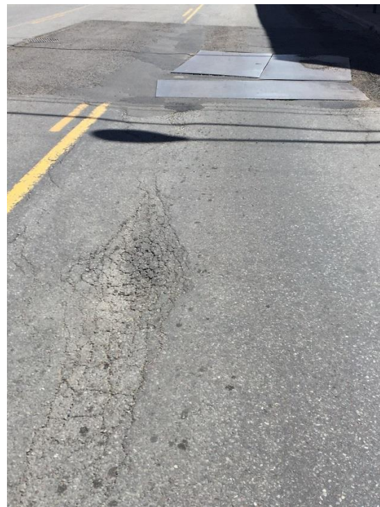
Photo 3 – Utility Trench Settlement, 300-Block of Railroad Avenue, Looking South
