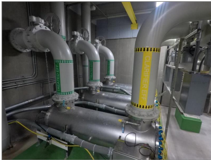
UV Disinfection Units
