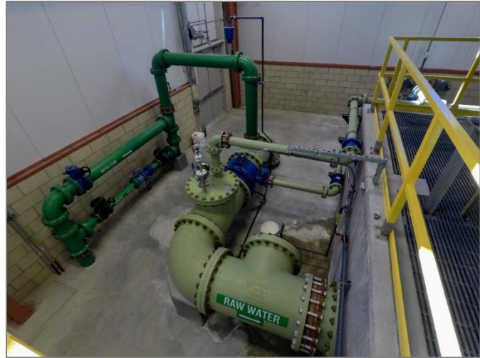
Pretreatment Chemical Injection and Jet Mixing Piping
