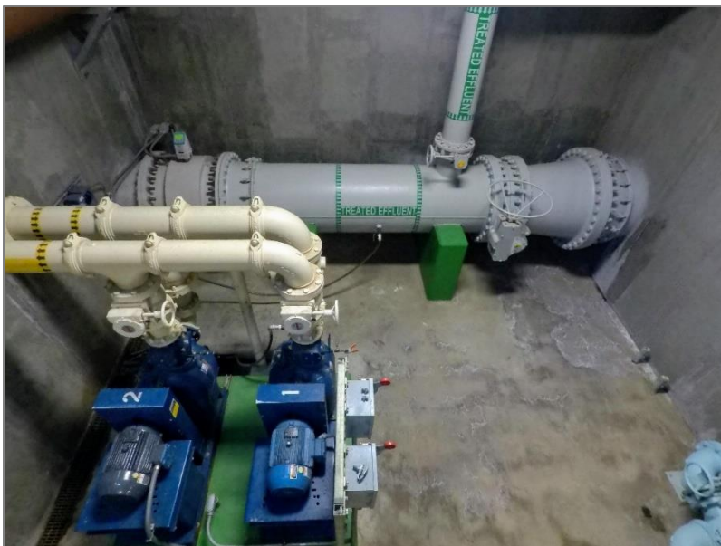
Treated Effluent Leaving the Disinfection Room
